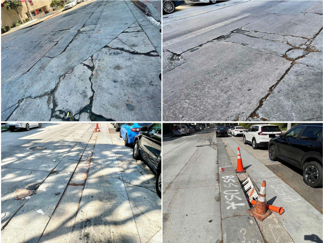
Figure 1. Tiverton Avenue pavement is in very poor condition, including numerous potholes and longitudinal grooves/ridges that can trap narrower bicycle and scooter tires, posing a serious safety threat.
