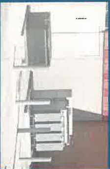
500KVA INTERIM SERVICE 08/05/2025
