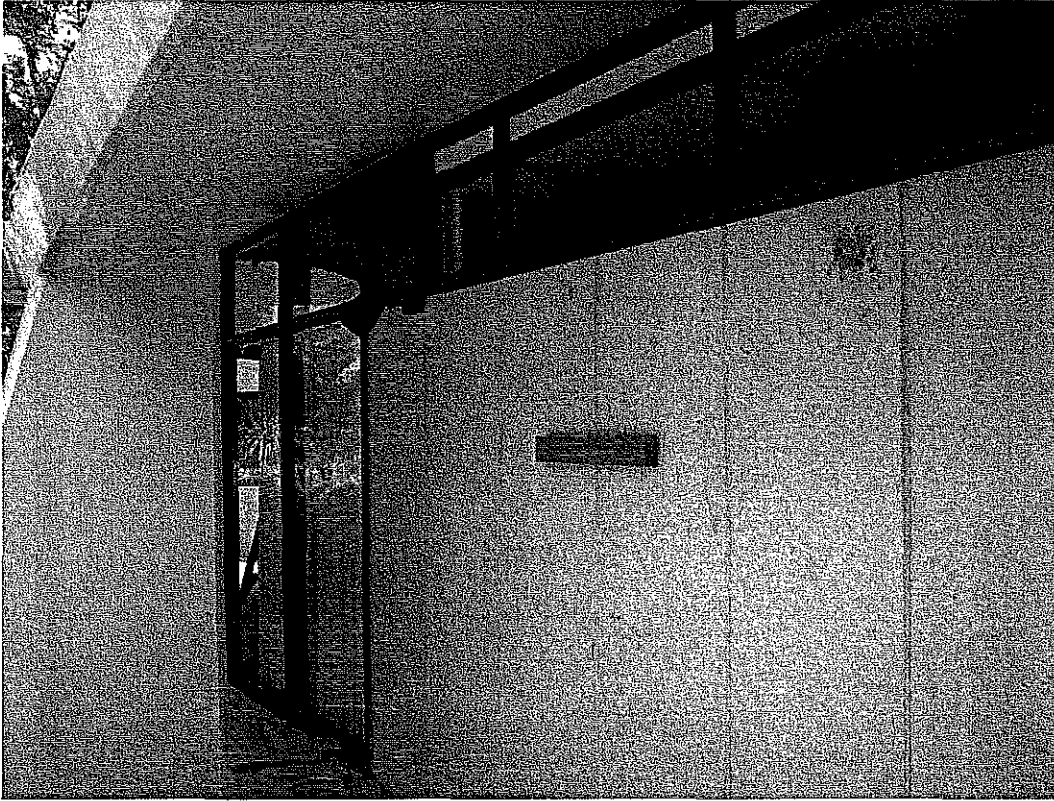
James F. Real Studio-Office, exterior partition wall, 77 Patrician Way (Photograph by Charles J. Fisher)
