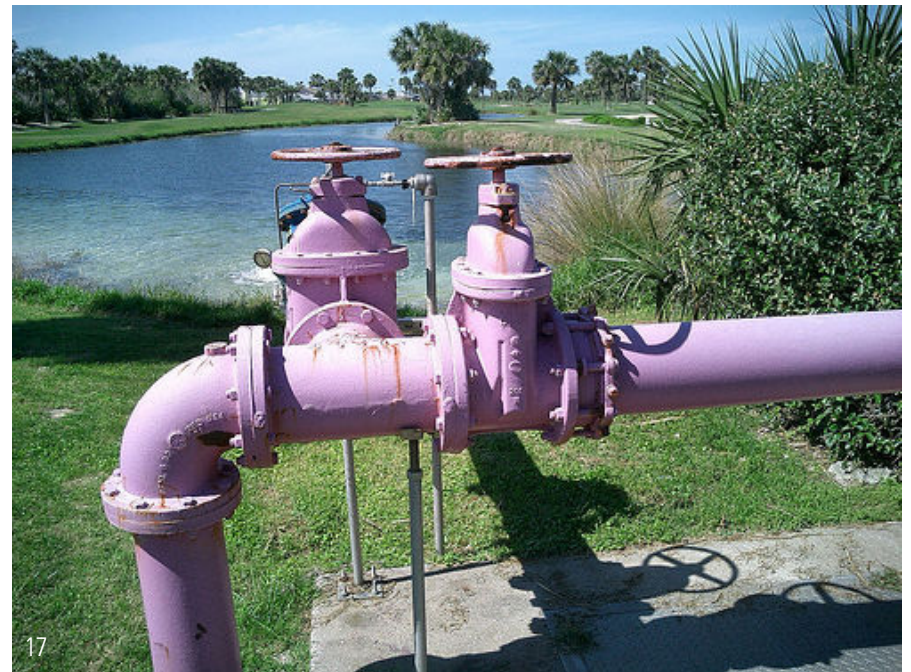
Purple pipe supplying reclaimed water
