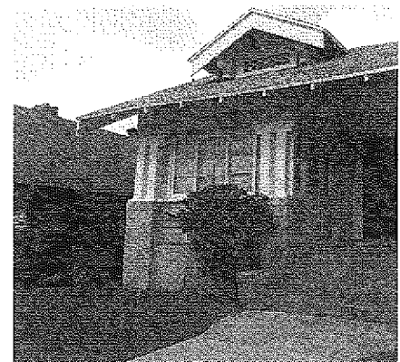
A portion of this porch has been enclosed in a manner that preserves the overall integrity of the porch components.
