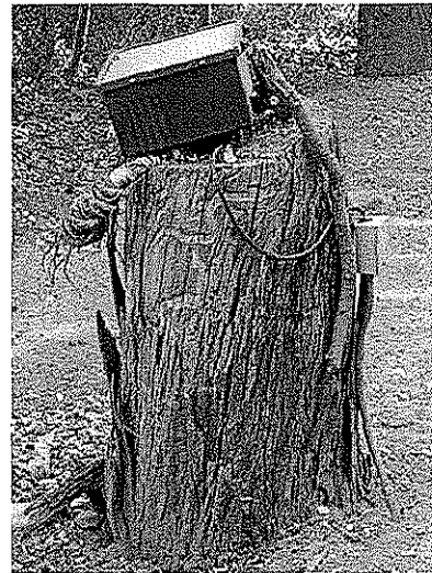
E030 - De-activated exterior flood light at Caracol Tower
