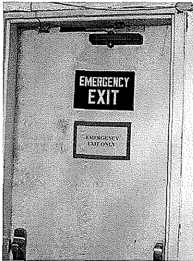
E019 - Administration area exit lacking proper illumination and signage.
