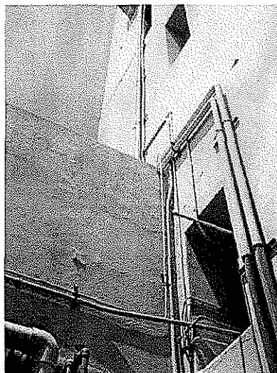
M003 - Piping from condenser; south face of Caracol Tower
