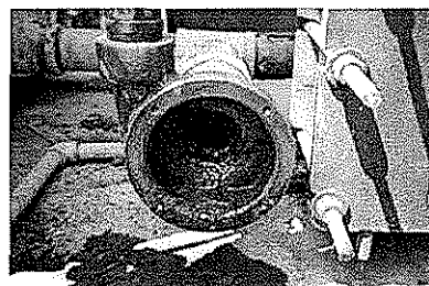
M002 - Back-up pump removed for service
