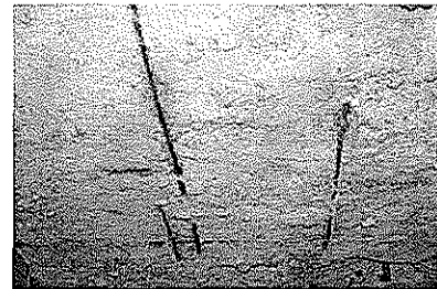
S001 - Rusted reinforcing bars below museum store
