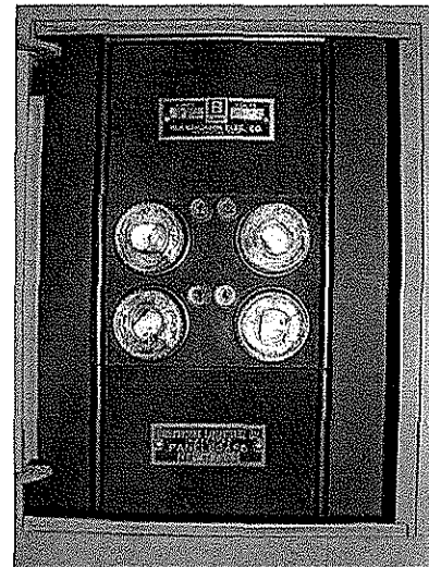
E002 - Boiler room fuse panel
