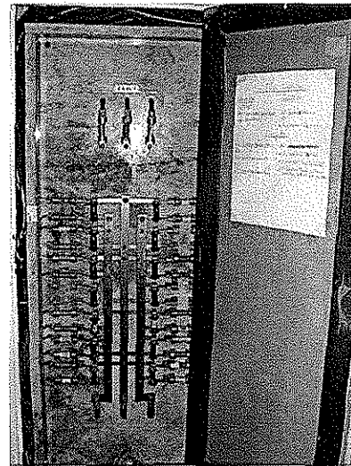
E016 - Plains Hall- marble panel showing multiple code violations
