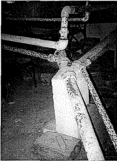
PO01 - Corroded galvanized steel water pipe
