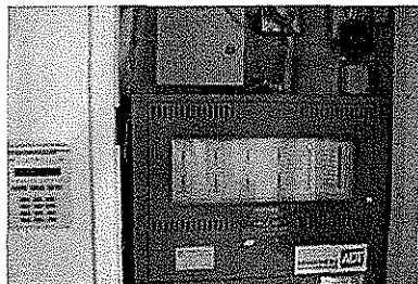
LS005 - Fire detection/communication equipment
