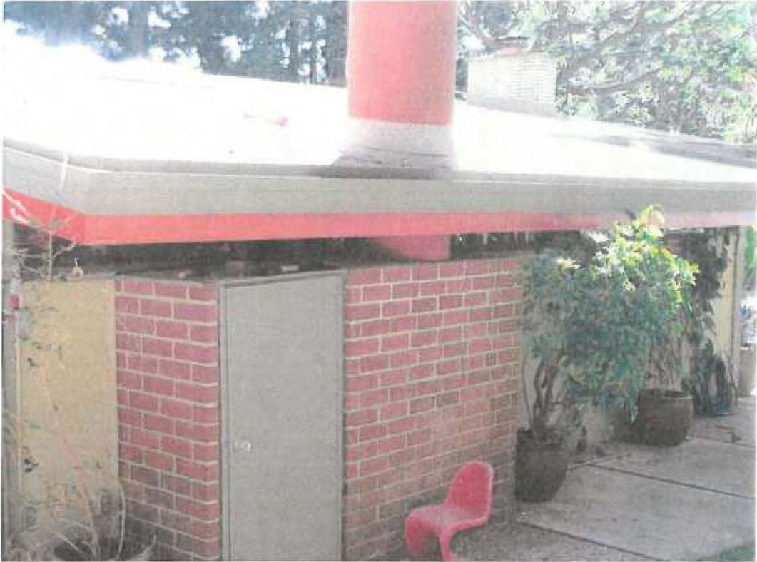
Zeiger House, 8941 Wonderland Park Avenue, den chimney, October 21, 2013 (Photograph by Charles J. Fisher)
