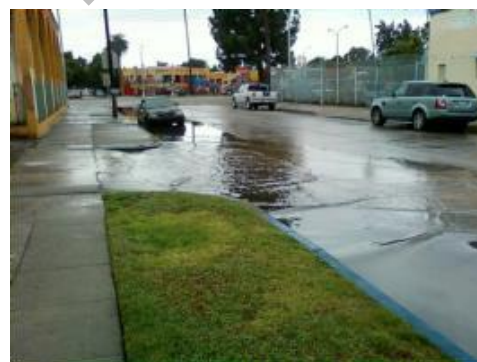
Figure 5-13 Existing Wet-Weather Flooding and Ponding Along the Proposed Vermont Avenue Project Site
