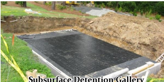
Subsurface Detention Gallery
