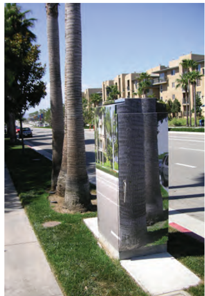
Mechanical equipment can be screened from public view by using innovative techniques.
