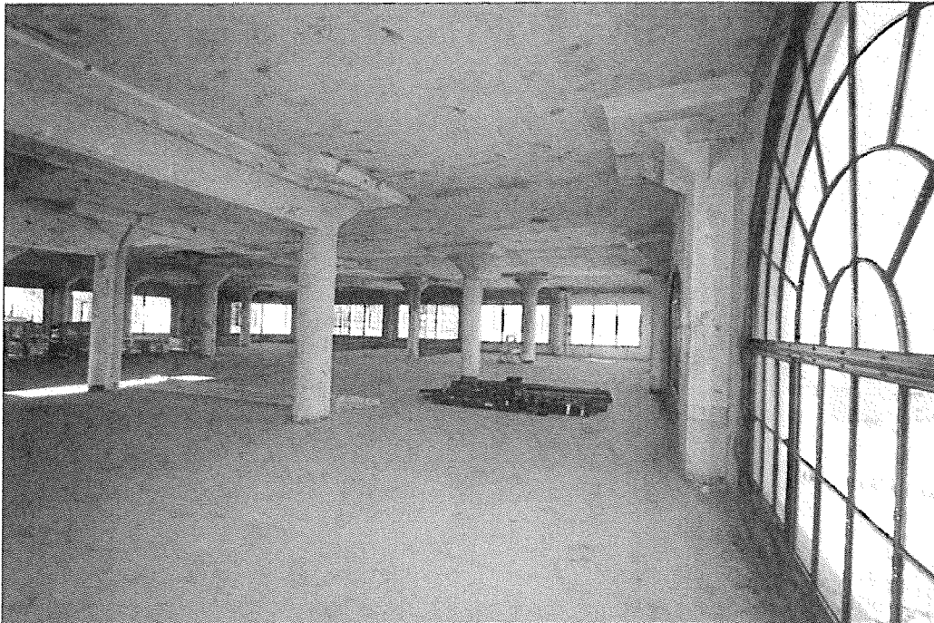
Photo 16: Maxfield Building, 819 S. Santee Street, interior view of typical upper floor open loft, during current adaptive reuse project (Chattel, 2014)
