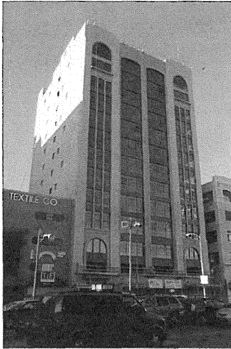
Photo 1: Maxfield Building, 819 S. Santee Street, exterior view northwest of east façade and south elevation, during current adaptive reuse project (Chattel, 2014)
