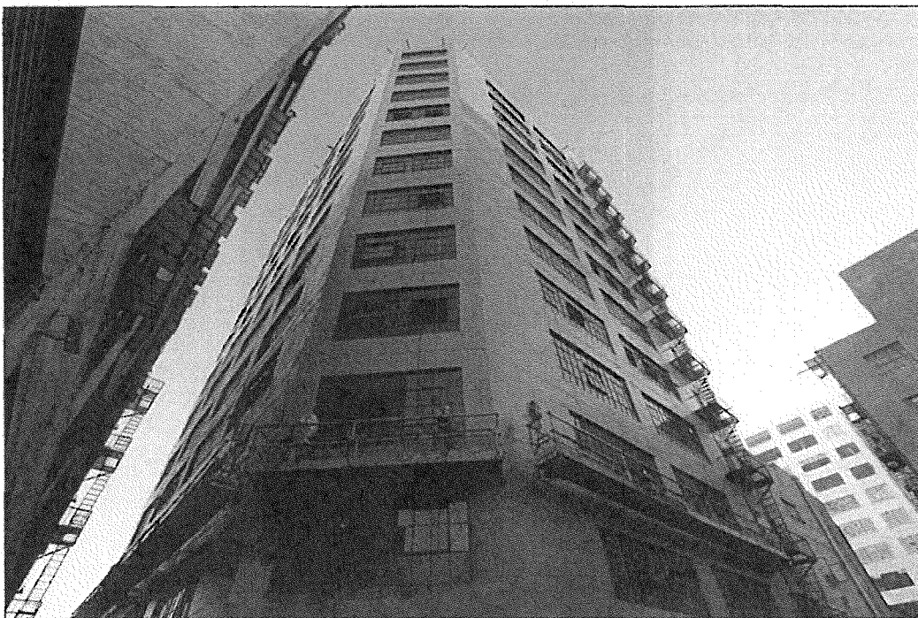
Photo 6: Maxfield Building, 819 S. Santee Street, exterior view southeast of north and west elevations, during current adaptive reuse project (Chattel, 2014)
