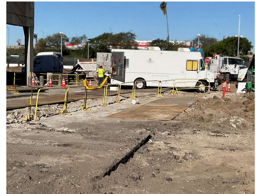
DWP field coordination along Pico Blvd. to support utility relocation & construction activities.
