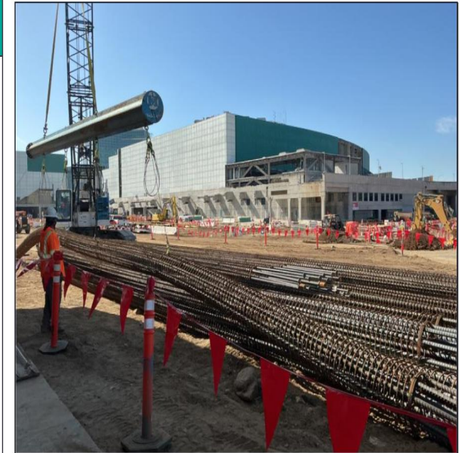
Major Milestone: Auger cast pile foundation work underway, drill rig installing piles - April 28, 2026
