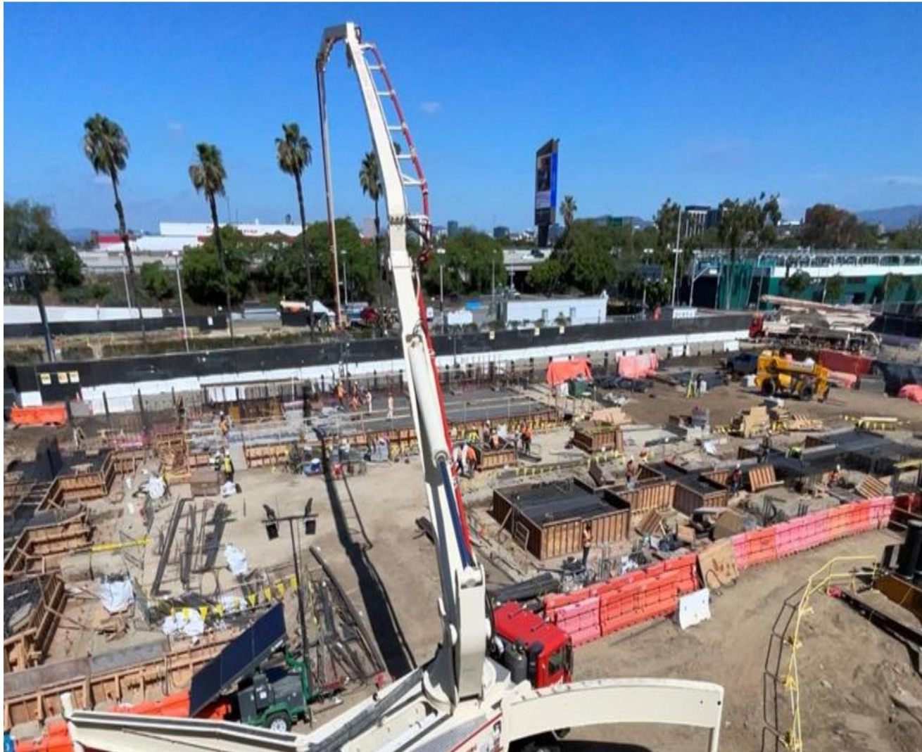
Auger cast piles completed (drilled and concreted in a single continuous operation); foundation grade beams and pile caps in progress - April 24, 2026
