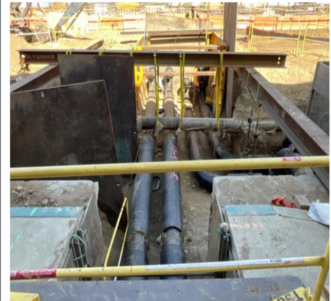
CHWS/R piping to Central Utility Plant (CUP) - April 29, 2026
