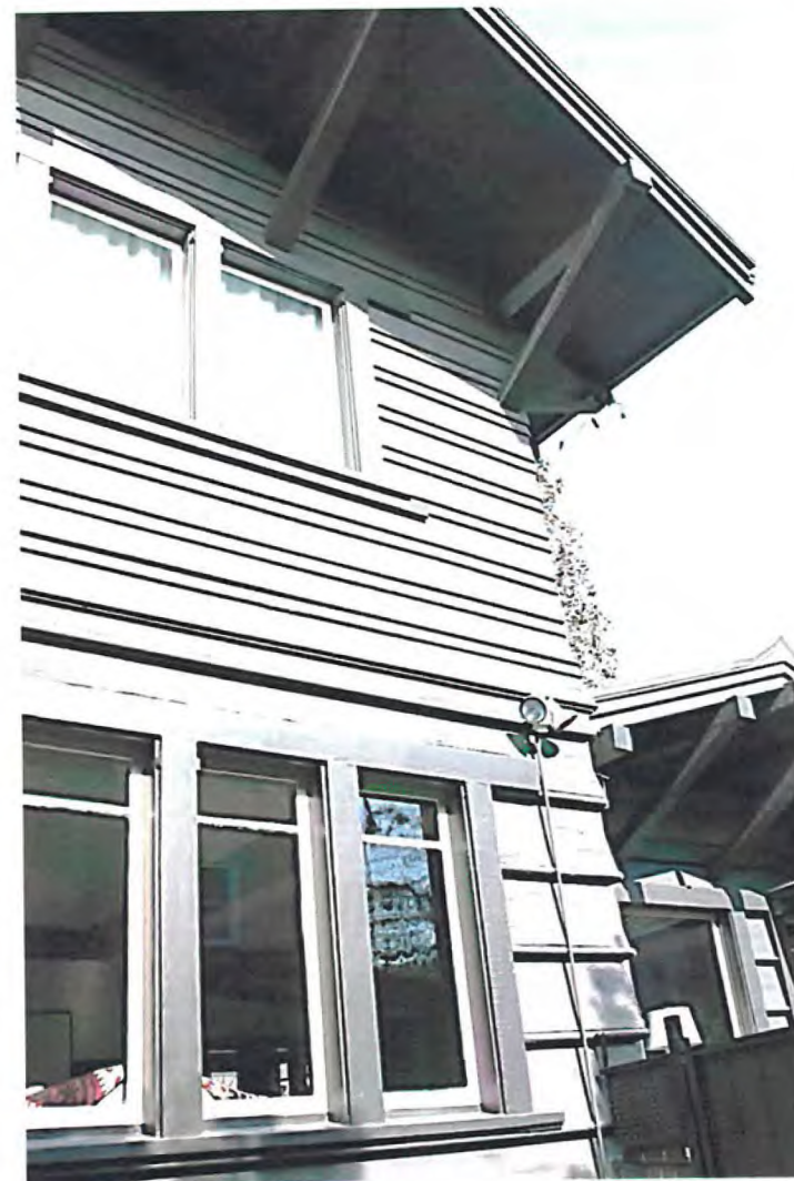
Detail: South elevation. Note variation in second and first story siding, view northeast.
