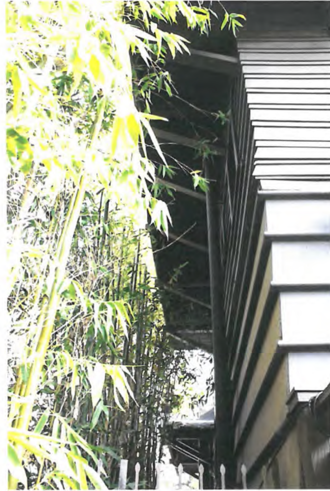
North elevation of residence: Brackets beneath deep eaves; differing types of siding clad first and second floor elevations. View east.
