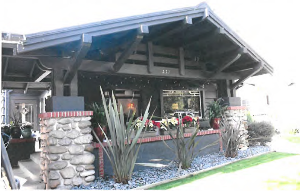
South & east wrapping porch: Original Craftsman, Airplane bungalow, with horizontal venting beneath deep eaves with brackets; steps at south and north, field stone/cement piers topped by brick band & wooden supports. View west.
