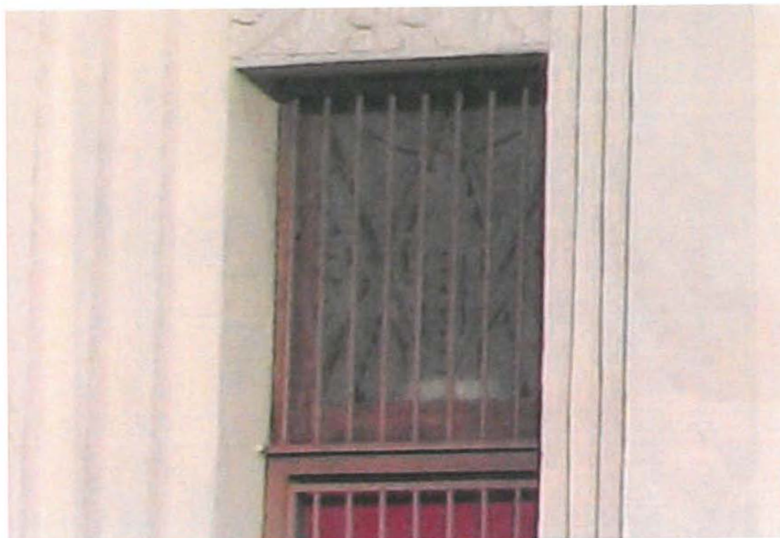
Redwine Building, etched transom window, 1618 N. Las Palmas Avenue, Feb. 5, 2015 (photograph by Charles J. Fisher)
