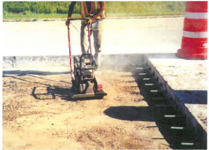
Figure 9. Recompaction of backfill immediately prior to placement of the new concrete surface course. Note that all other necessary preparation work has been completed, such as the dowel bars already having been drilled and installed.
