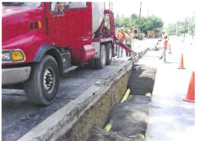
Figure 10. Placement of flowable backfill in a utility cut. Note that the flowable material is self-leveling, with the top of the backfill being placed to the base of the existing adjacent concrete slab [Photo courtesy of the Cincinnati Ready-Mix Concrete Company].
