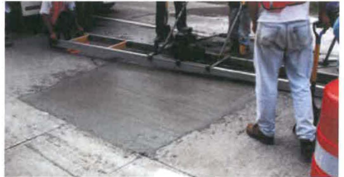
Figure 15. The new concrete surface course of a utility cut restoration being finished by a vibrating screed. Note that the surface is being finished perpendicular to the centerline because the utility cut length is less than 10 ft (3.0 m).
