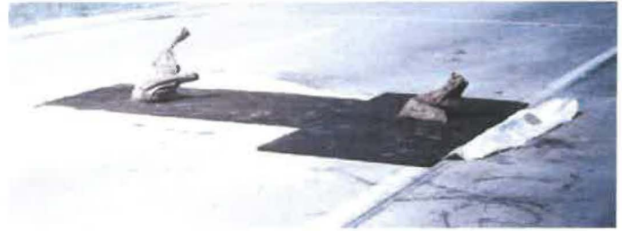
Figure 19. Insulation mats placed on top of polyethylene sheets to encourage a relatively quick strength gain.
