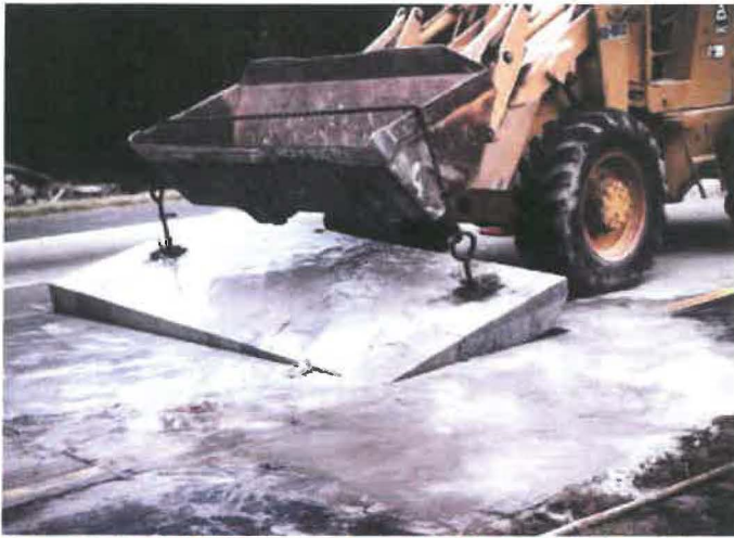
Figure 7. Partial slab removal using a lift-pin and chain lift-out method with a front end loader.
