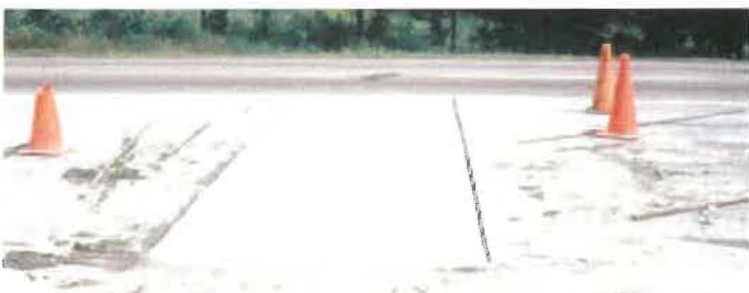
Figure 18. Proper application of white-pigmented membrane-forming curing compound. Note that the surface of the repair area is as white as a sheet of paper.
