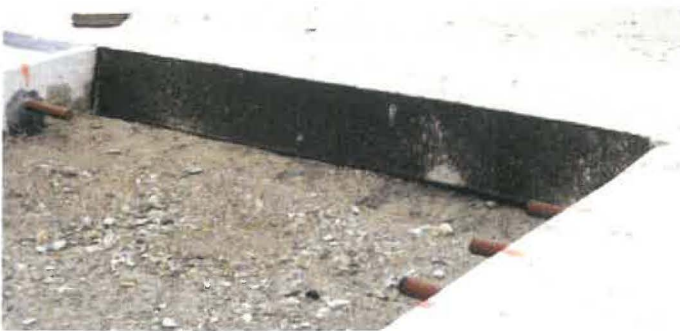
Figure 13. Fiber-board bond breaker placed along the longitudinal joint between the existing pavement and the utility cut section because the utility cut section is not longer than one slab.
