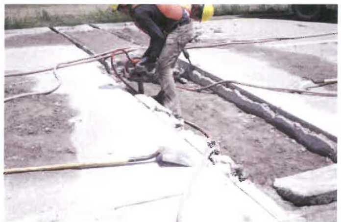
Figure 6. Breakup of a utility cut area in a concrete pavement thinner than 7 in. (175 mm) after sawing the perimeter to a depth of about one-third of the slab thickness and making two transverse full-depth kerf cuts several inches from the transverse boundaries (note the remaining slab with kerf cuts in the background) to further aid in removal of the section. Also note that the saw-cut area is being removed with light jackhammers to obtain a slightly-tapering-inward joint face on the transverse joints, without undercutting the slab.
