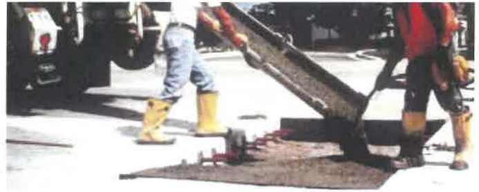
Figure 14. Proper concrete placement operations, with the concrete being discharged directly onto the subgrade/subbase inside the utility cut restoration area and a hand vibrator being used to ensure proper consolidation in the repair area and, especially, around embedded steel.
