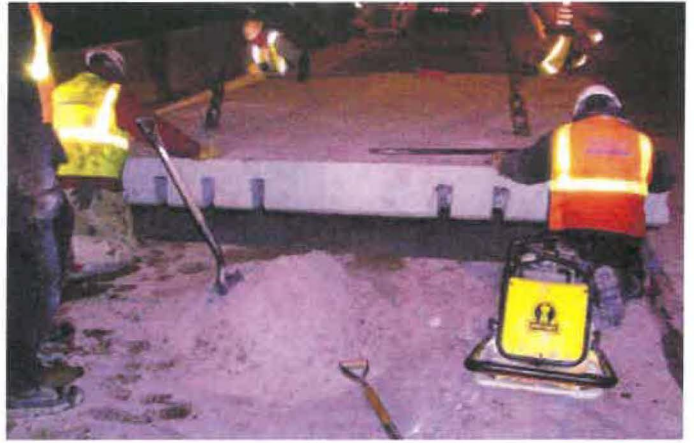
Figure 20. Positioning of a precast panel during a utility-related repair in a nighttime closure [Photo courtesy of The Fort Miller Co., Inc.].
