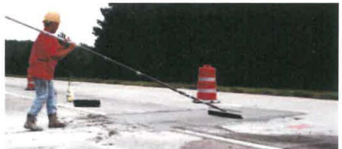
Figure 17. Texturing of a utility cut surface using a broom. Note that the curing compound is sitting nearby so that it can be applied as soon as possible.
