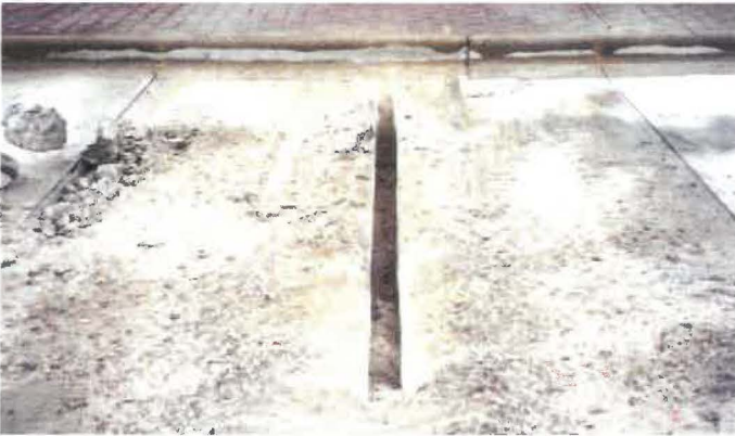
Figure 5. A pressure relief cut made using a carbide toothed wheel saw (kerf saw) down the middle of a utility cut to aid in removal of the section.
