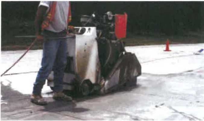
Figure 4. Diamond-bladed saw making perpendicular, straight cuts around the perimeter of a utility cut.
