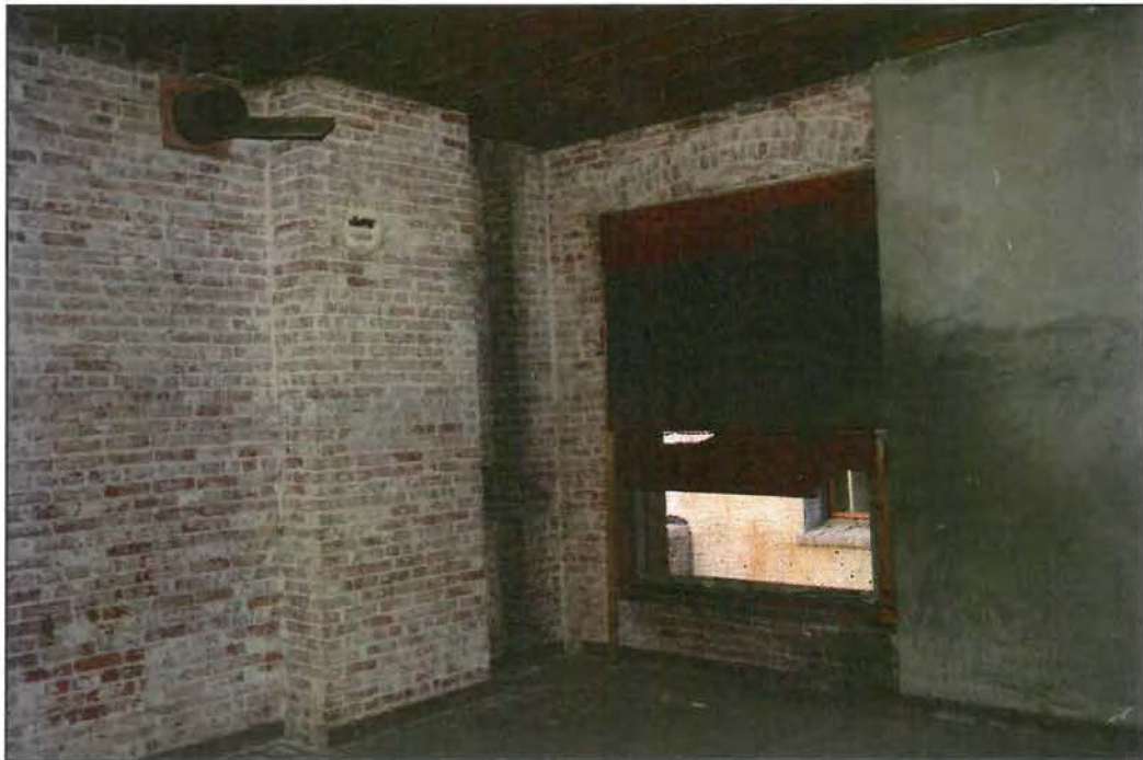
Figure 101: Interior view, exposed brick and windows in need of repair (Chattel 2015).
