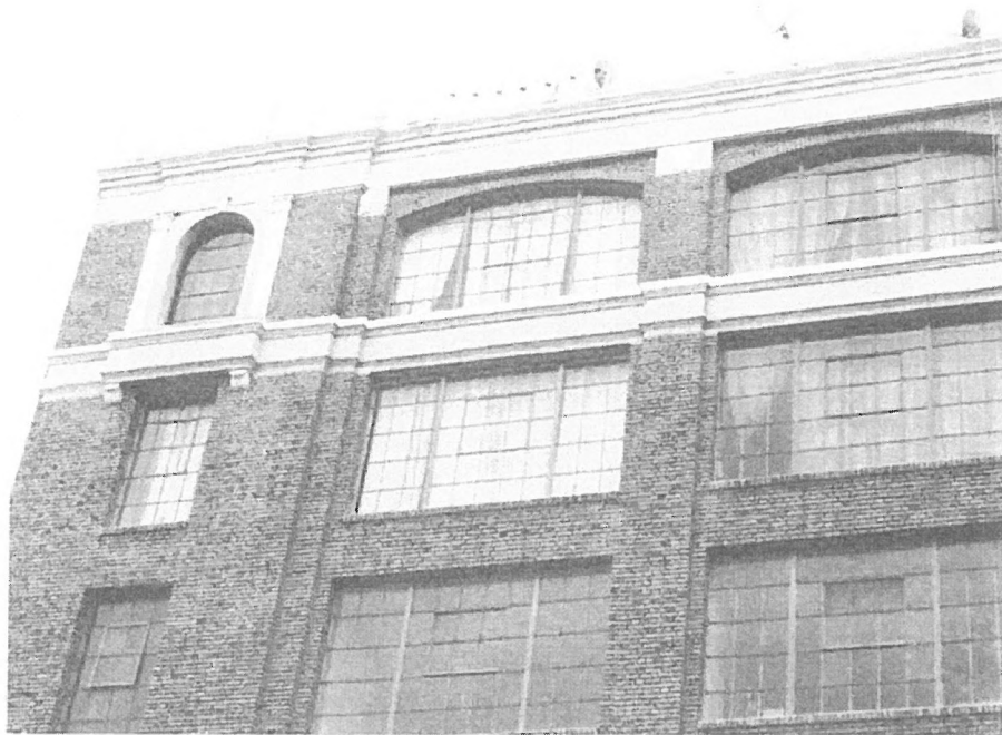
Upper story, modest neoclassic detailing adds stylistic identity to a manufacturing building, typical of the early work of W. Douglas Lee.
