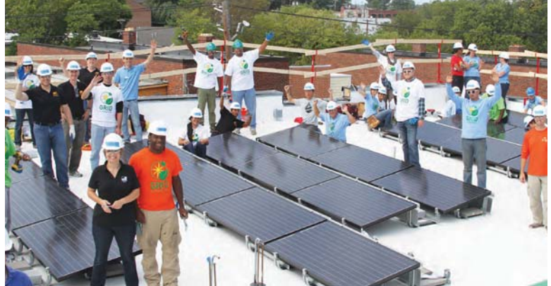
An aggressive commitment to rooftop solar installations in Los Angeles will expand the local economy, accelerate the transition to clean energy, and lead to dynamic job growth.
