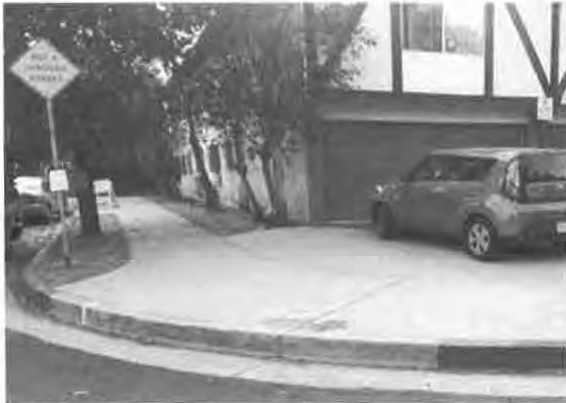
Curb Ramp Needed
