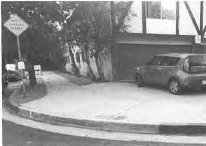
Curb Ramp Needed
