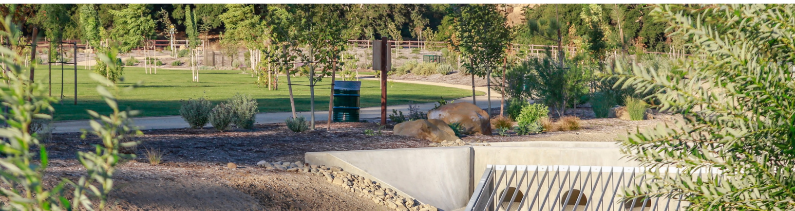
Stormwater infrastructure in Chatsworth Park South.
