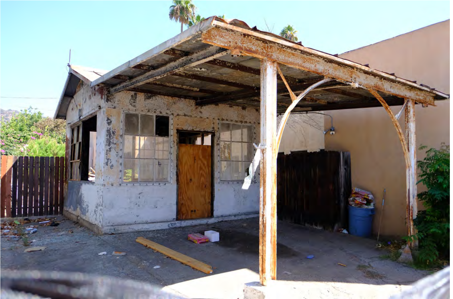
Jay Risk Standard Oil Co. Service Station. View northeast. Photographed after the owner started to disassemble the building. (Sullivan 2022)
