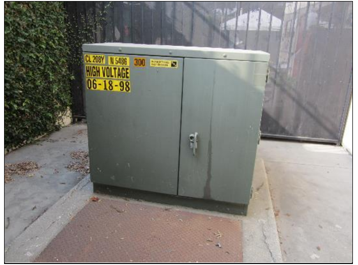
20. Pad-mounted electrical transformer on the subject property.
