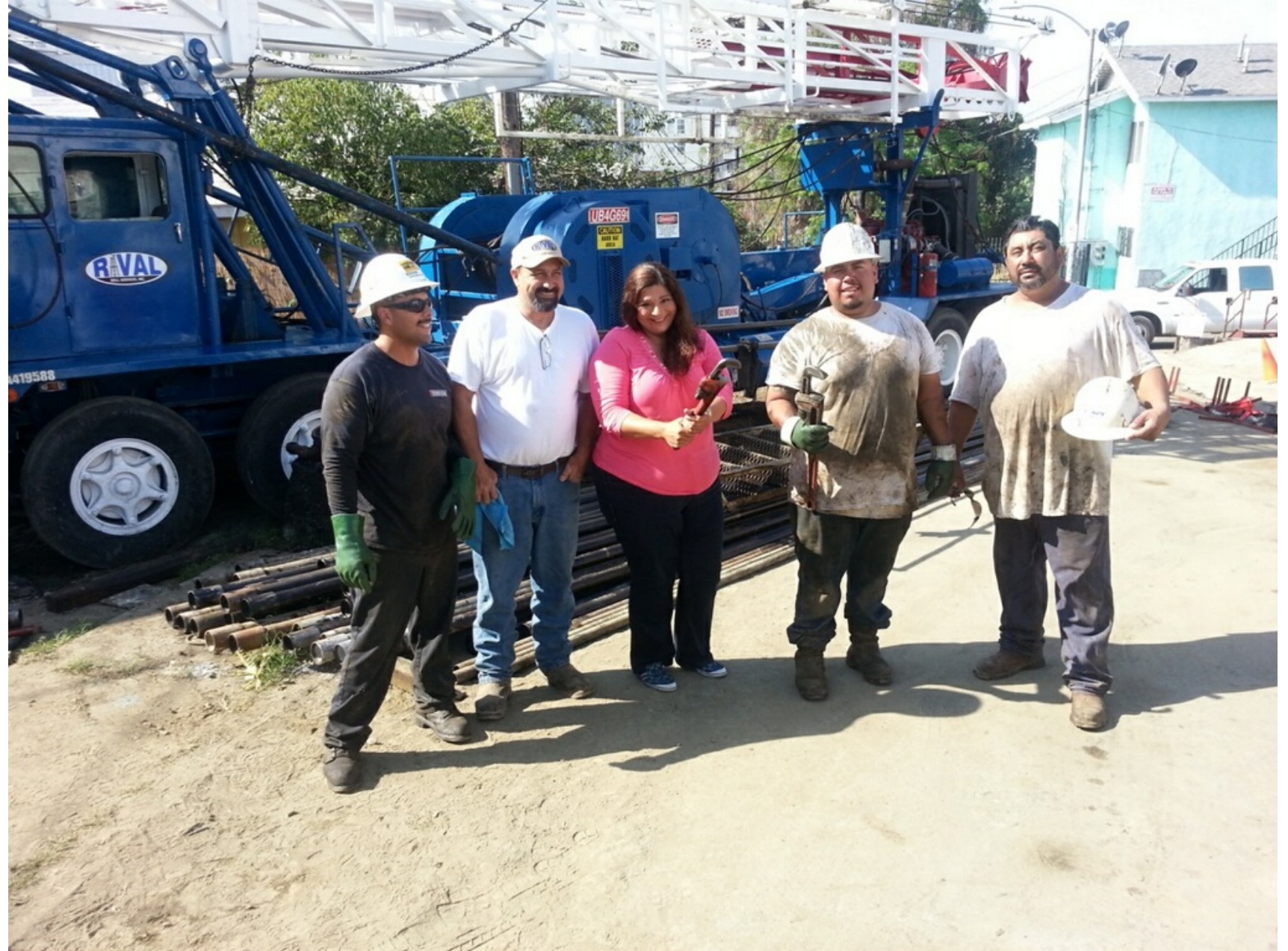
Photo From DeSmog: Rosalinda Morales (center) with the contractors capping an orphan well on Firmin Street. Credit: Courtesy of Rosalinda Morales
