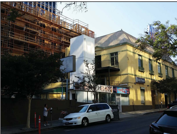
View 5: Looking northwest on Harvard toward under construction residential development and commercial uses.
