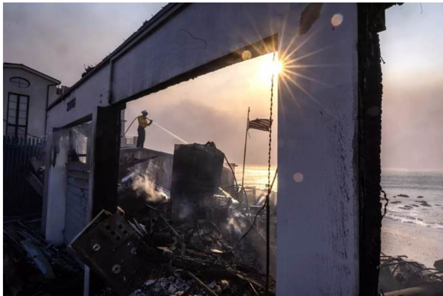
Beachfront homes are devastated by the Palisades fire on PCH in Malibu. (Brian van der Brug/Los Angeles Times)
