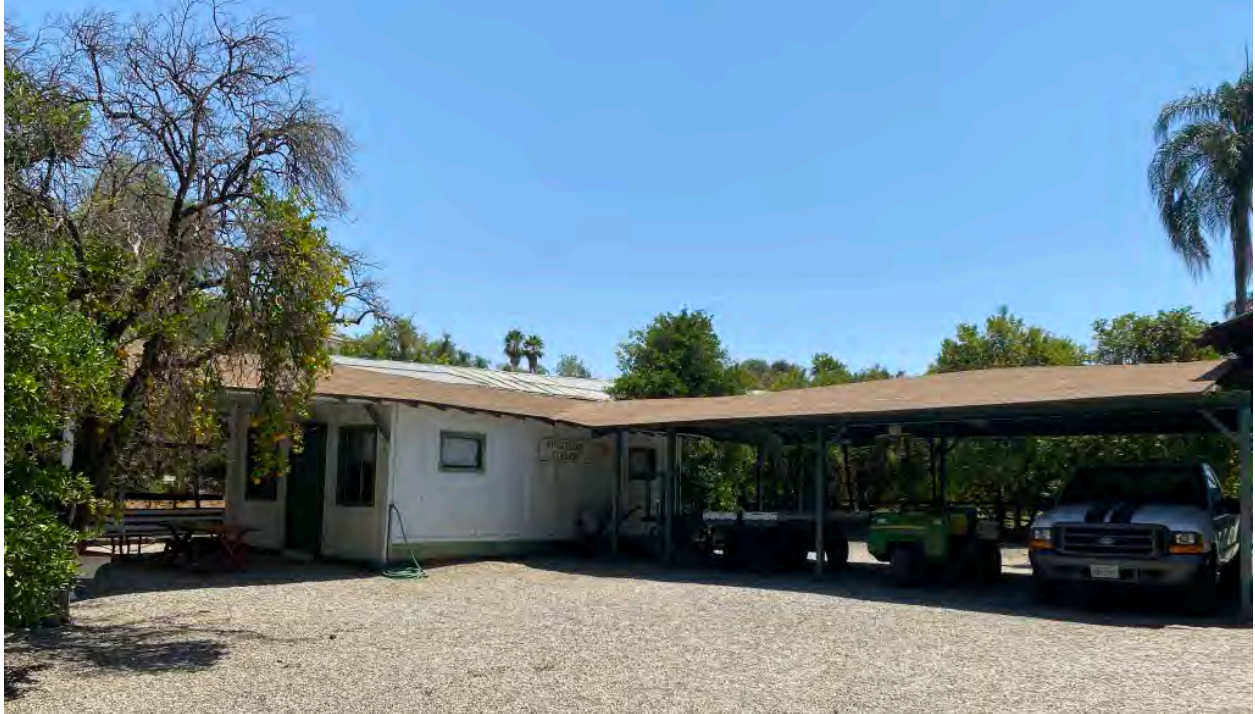
Figure 20: July 2022 view of train station on Project Site looking southeast from multi-purpose building.
