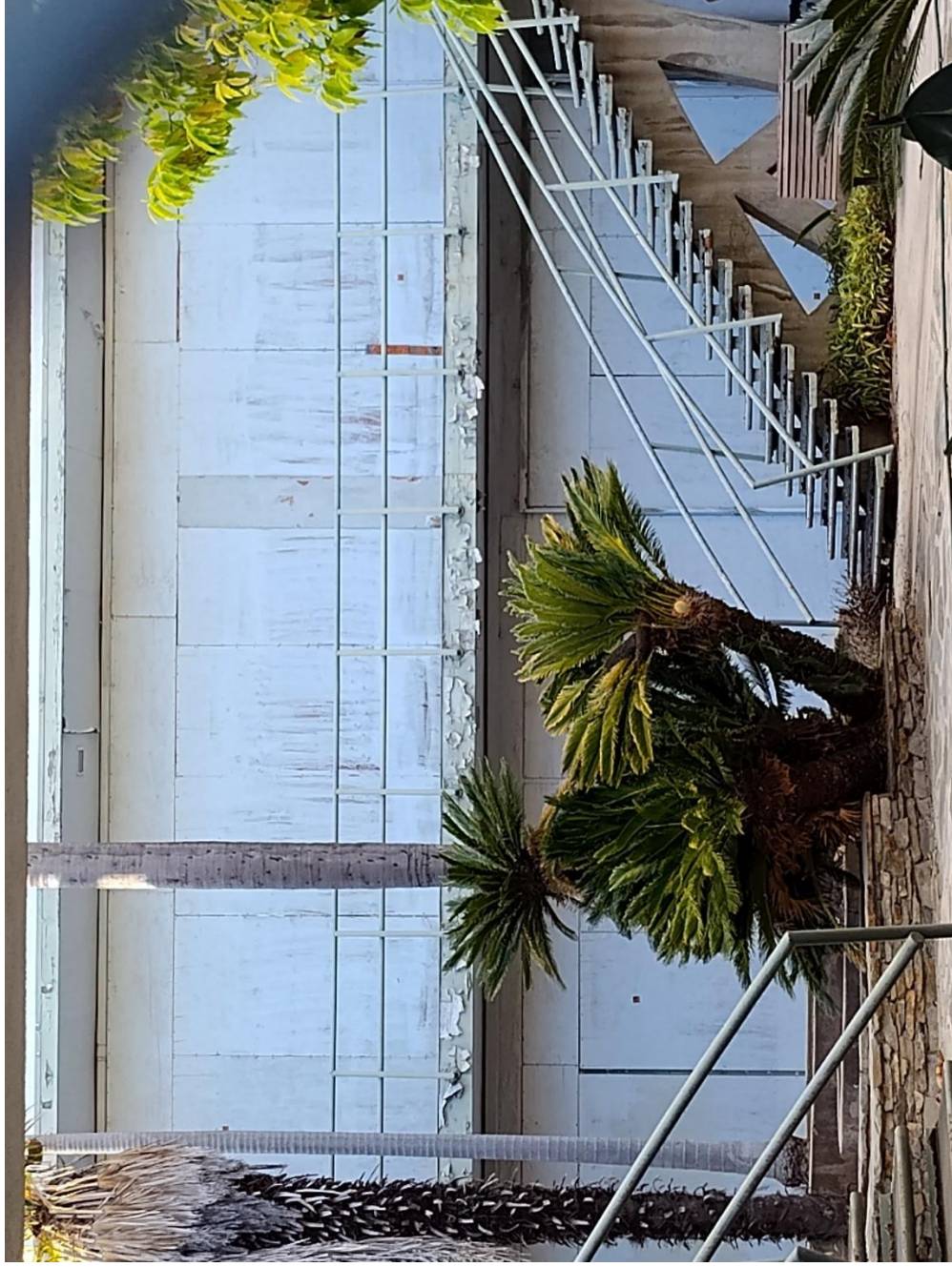
1. Court Yard showing flaking paint and deteriorated conditions, 04-13-2026
