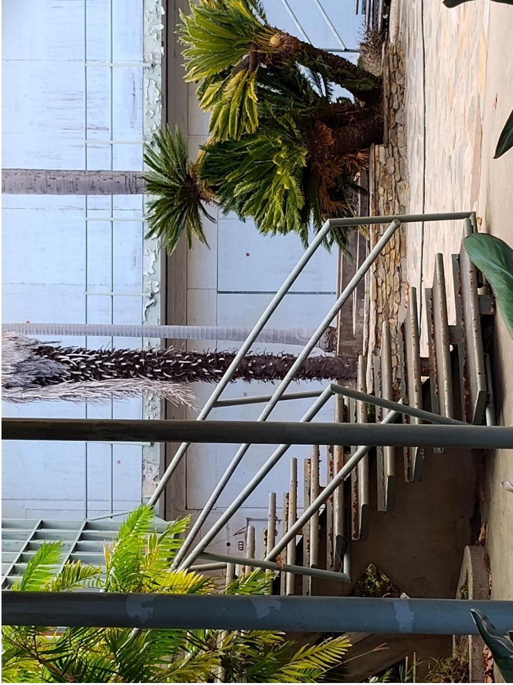
2. Court Yard showing deteriorating staircase and walkway, 04-13-2026
