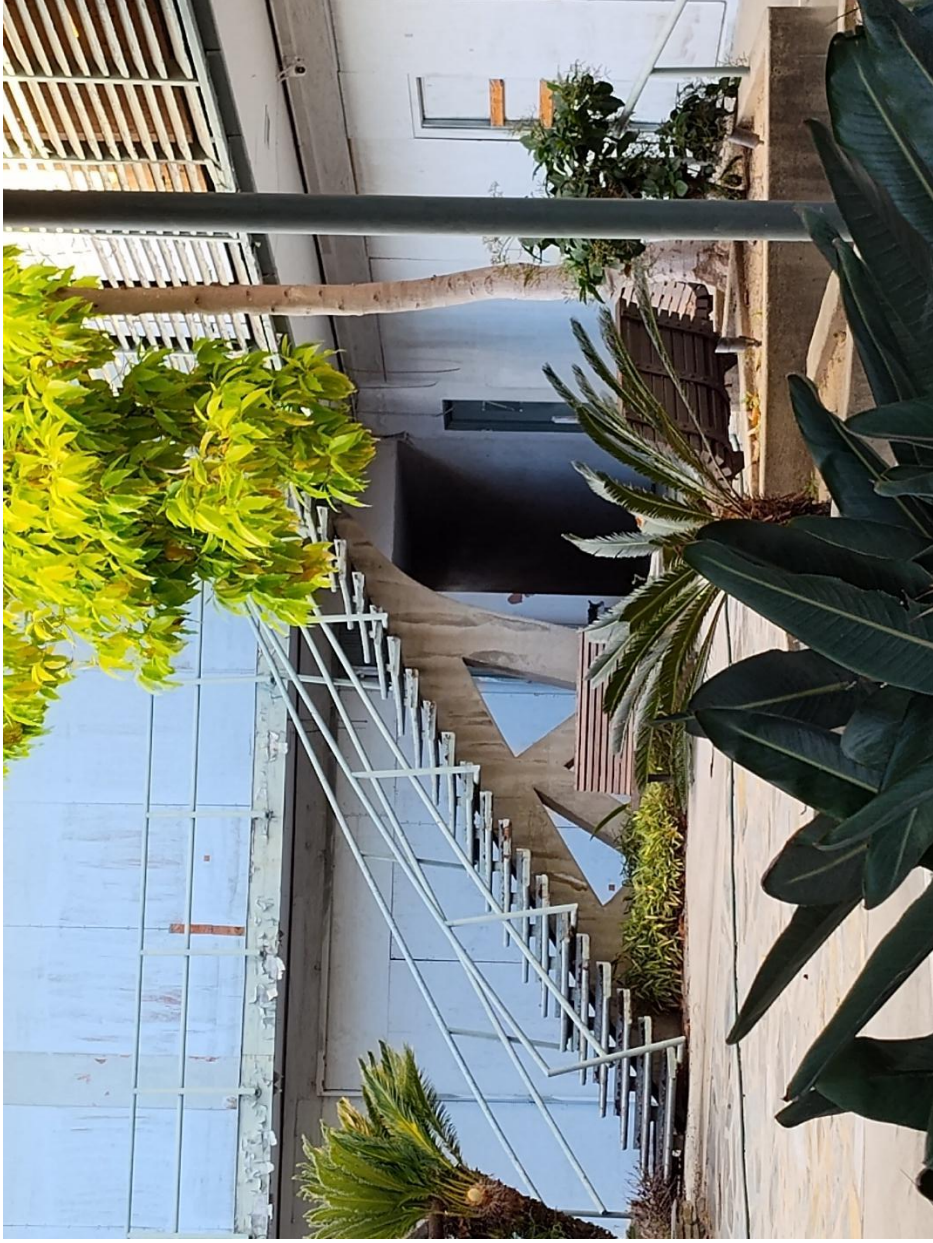
3. Court Yard showing deteriorating staircase and walkway, 04-13-2026
