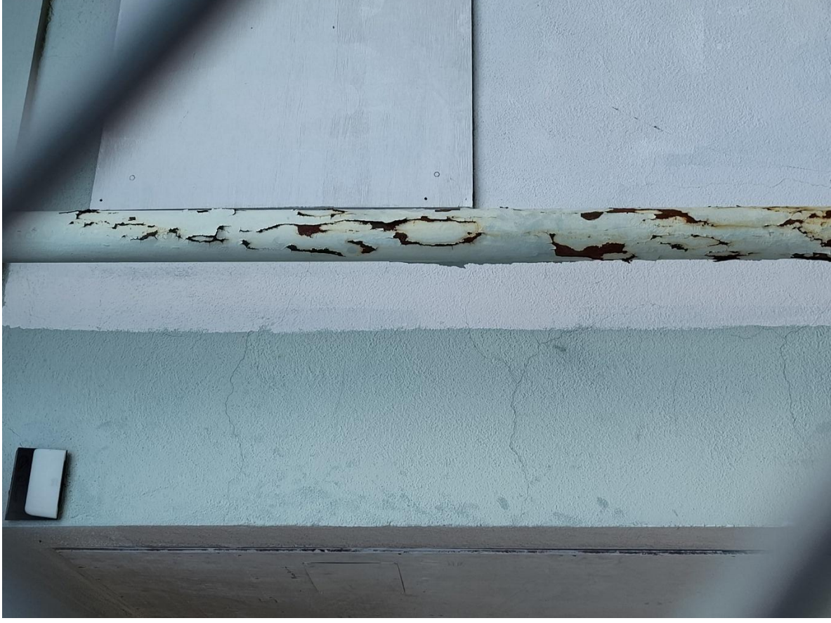
7. Flaking and Rusting steel column, 04-13-2026
