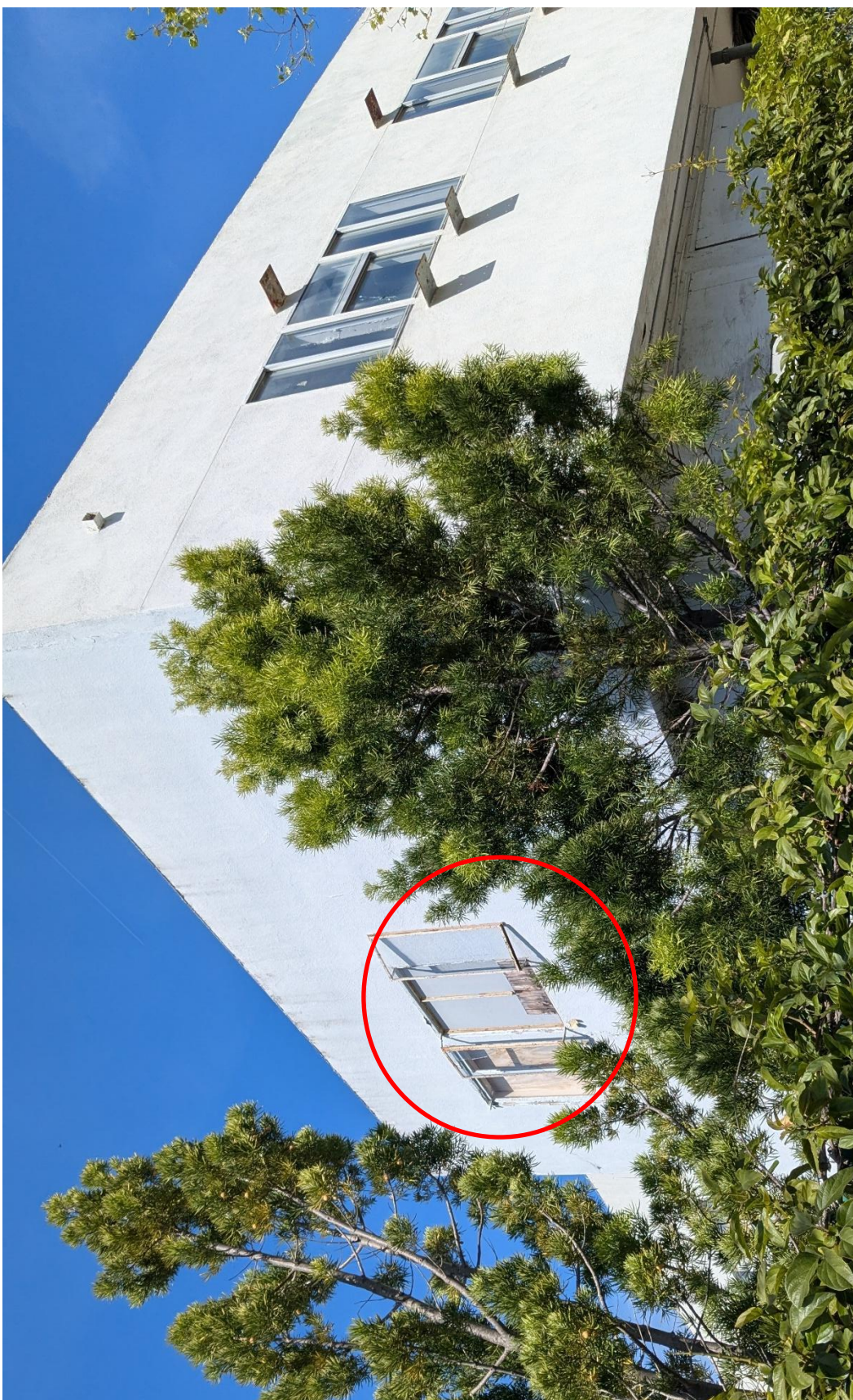
5. West Side of South Wing showing Open Windows, 03-10-2026 (Circled in red)
