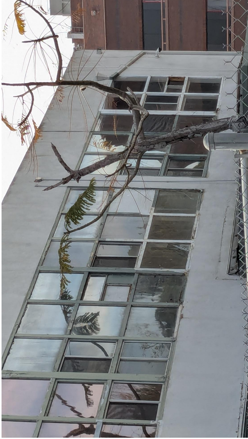
2. North Side showing deterioration, 02-03-2025
