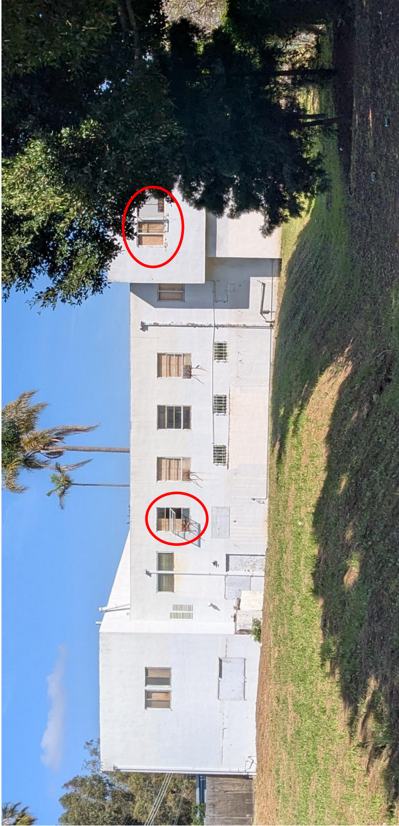
4. West Side showing open windows, 03-10-2026 (Circled in red; one year later from Photo 1)
