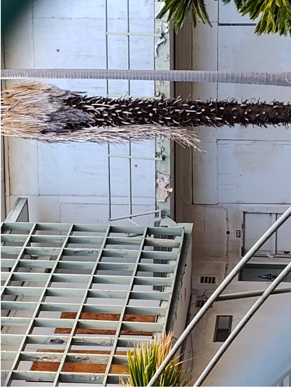
6. Court Yard showing flaking paint, 04-13-2026
