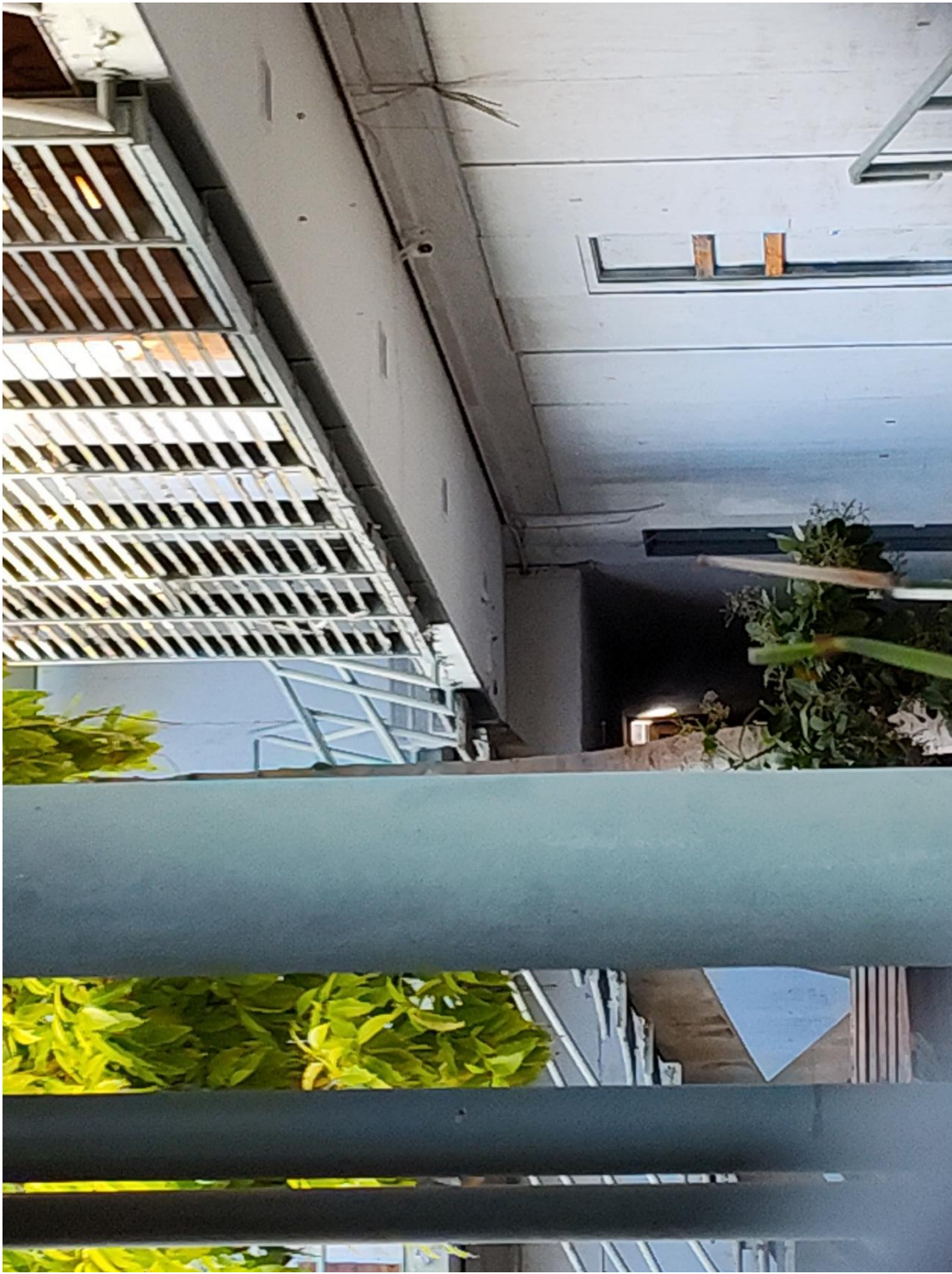
5. Court Yard showing deteriorating louvers, 04-13-2026
