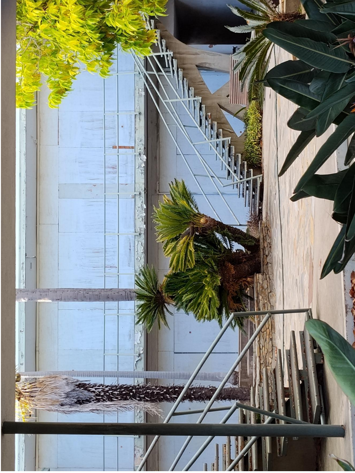
4. Court Yard showing both deteriorating staircases, 04-13-2026
