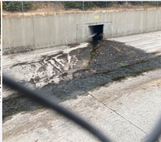
Dark muck flowing into the River
