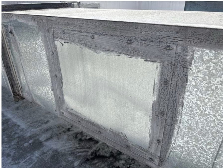
HA 7 - Grey HVAC Duct Mastic
