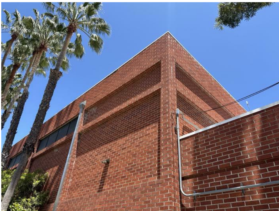
Assumed ACM - Upper Roofing Materials
