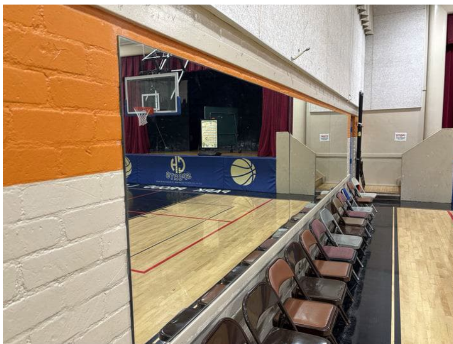
Assumed ACM - Mirror Mastic
