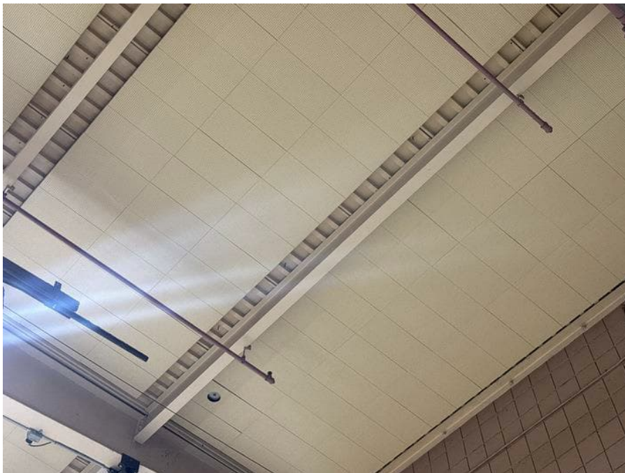
Assumed ACM - Acoustic Ceiling Tiles
