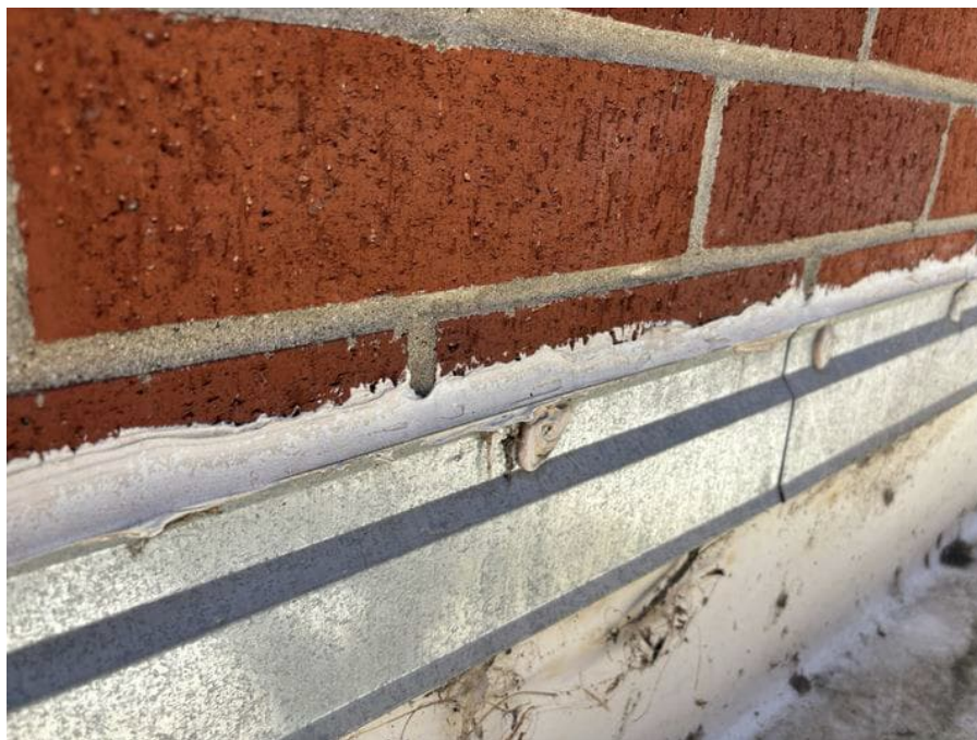
HA 9 - White Wall Seam Caulking
