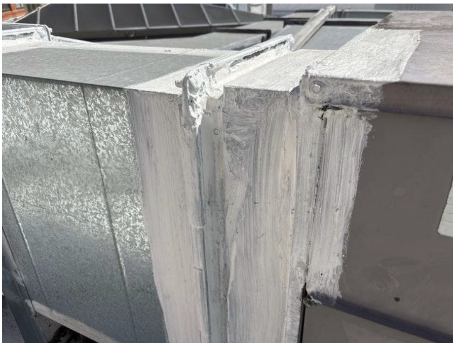
HA 6 - White HVAC Duct Mastic
